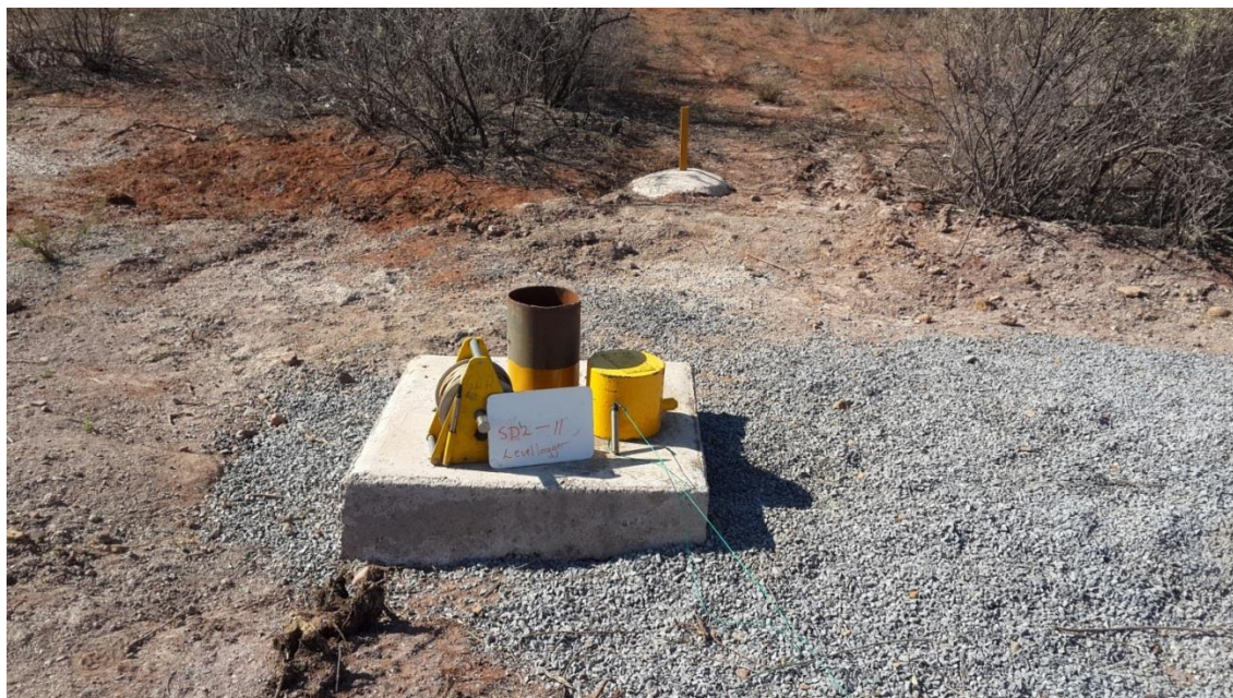
Figure 49: SD2-11 Installed Water Level Logger
